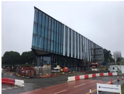
Caption: August 2022. Progress on Aberdeen's £40 million Bio Hub project with curtain walling now complete, final cladding being installed and internal fit out progressing to plan.
